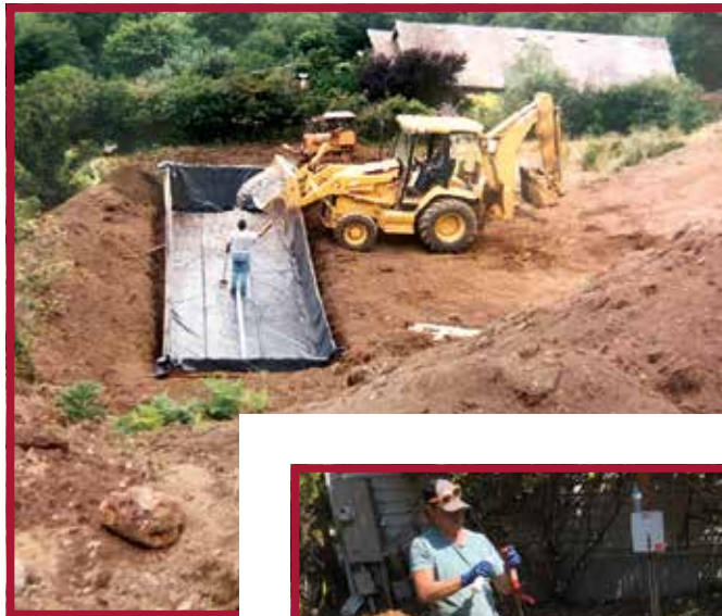
◀ Installation of sand filter in a local development, with Pat McVay operating a Caterpillar 416C backhoe and Jay Hopkins assisting. A CASE 450 dozer is shown in the background.
