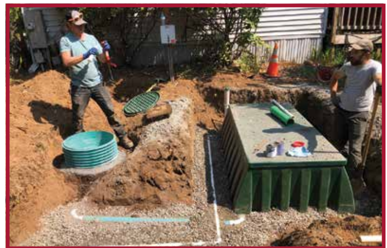
✔ An Orenco Systems AdvanTex AX-RT unit being installed by Kevin Cain (left) and Johnes Winn.
