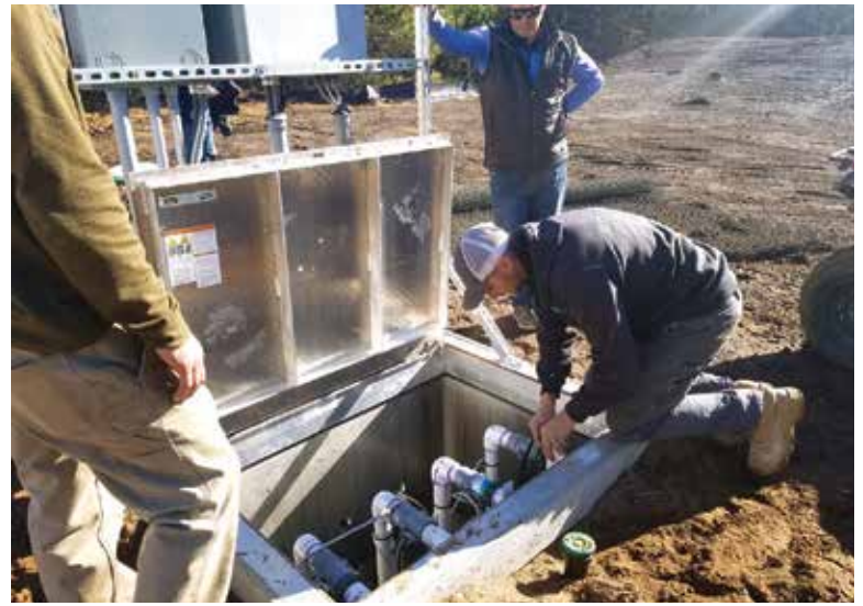
▲ Brian Koski of Septic Check, adjusts a component on a commercial system (Infiltrator ECOPOD) at the University of Minnesota Cloquet Forestry Center.
